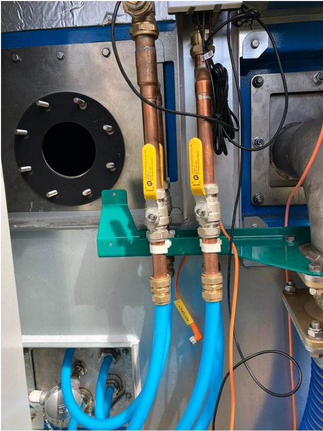
Piping and valves
