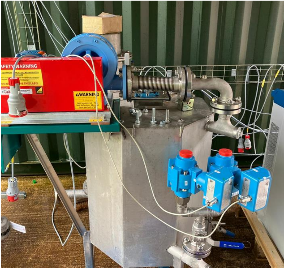
Biogas treatment pod
