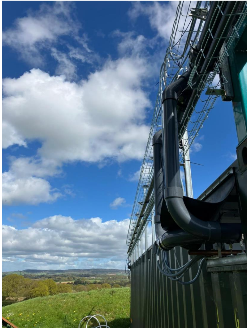
Anaerobic digester unit for biogas production
